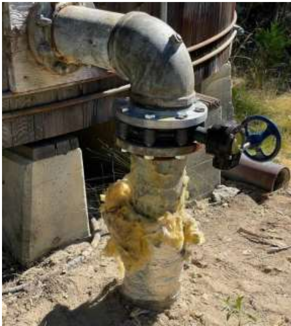
Figure 3: DPH water tank isolation valve
