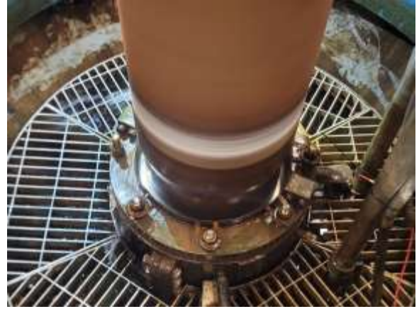
Figure 2: Tulloch Powerhouse Unit 3 packing
