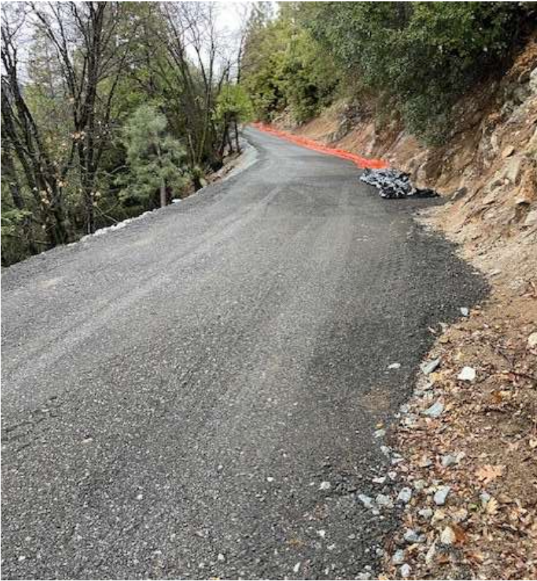
FEMA Site 6 Donnells Road Large Washout
