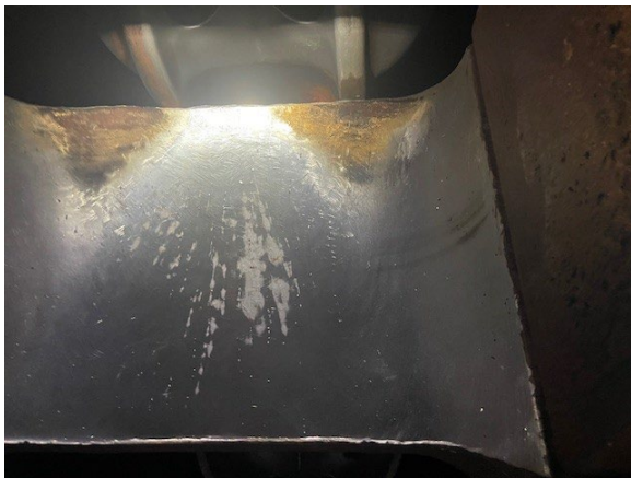
Figure 1: Wear on Donnells Deflector No. 5
