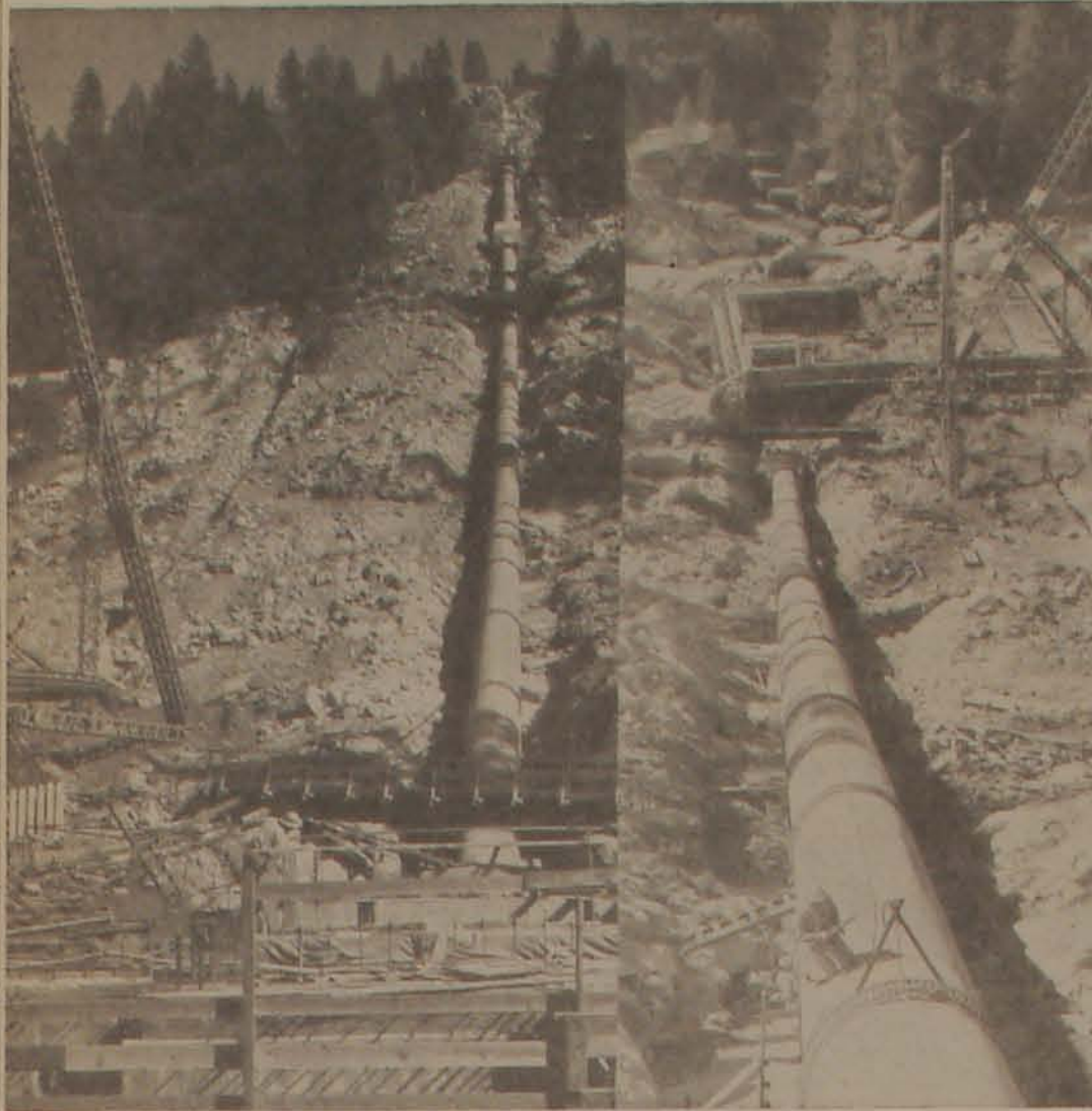
THE UP AND DOWN OF IT —Here are two views of the penstock, or water pipe, which carries the water out of the tunnel from Donnell's Reservoir, down a 1,200 foot drop to the powerhouse. Taken during construction last
